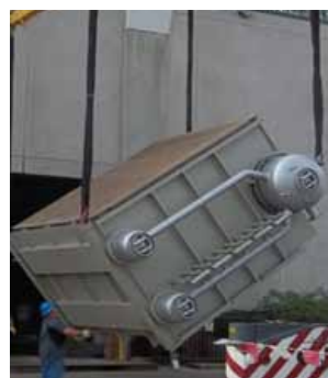
Pepco Cogeneration Plant
